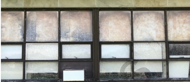
Exterior - Energy inefficient and aging infrastructure
